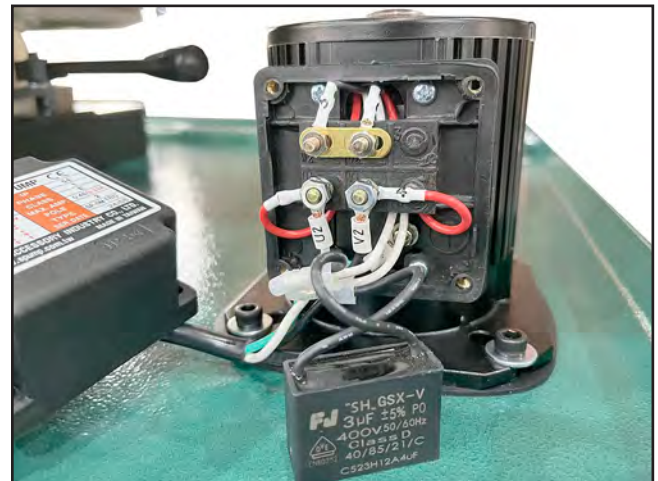
Figure 1. Pump motor wiring.
