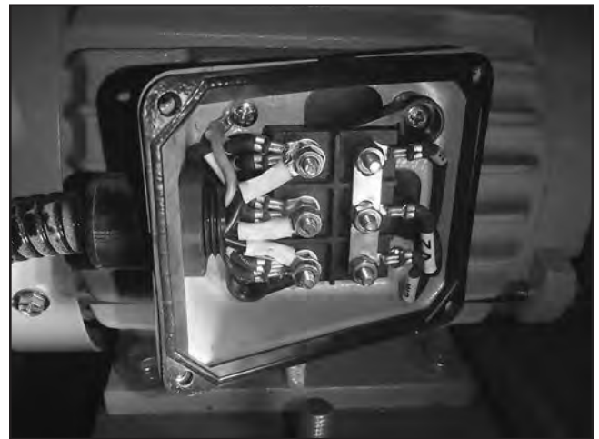
Figure 50. 220V feed motor wiring.
