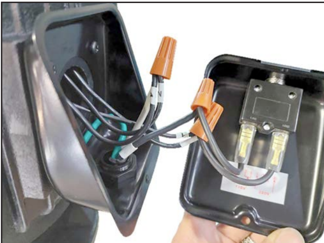
Figure 84. Main motor junction box wiring (110V).
