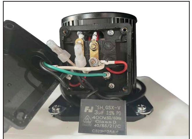
Figure 87. Pump motor junction box wiring (110V).
