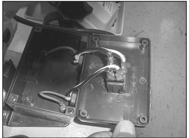
Figure 43. Switch wiring rear view.
