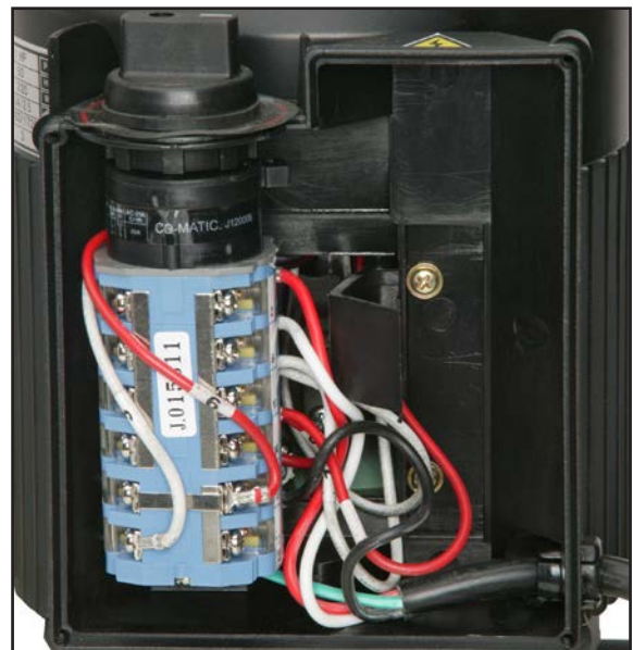
Figure 26. Motor switch and capacitor (front view, G1095).
