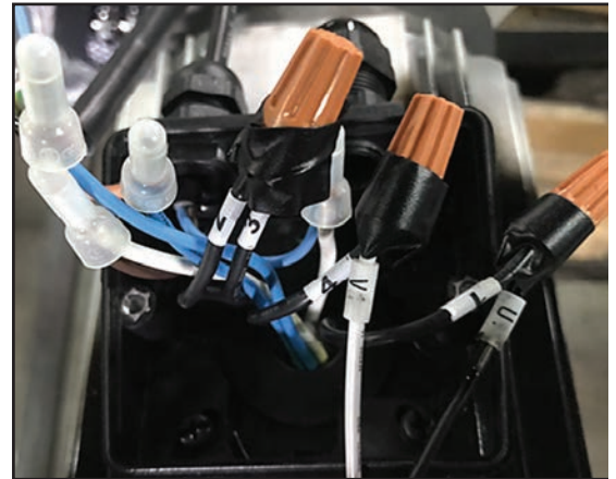
Figure 11. Main motor wiring.
