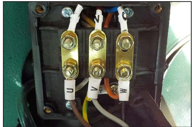
Figure 16. Pump motor wiring.
