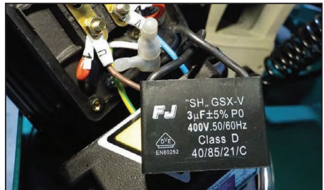
Figure 2. G0613 pump motor capacitor.
