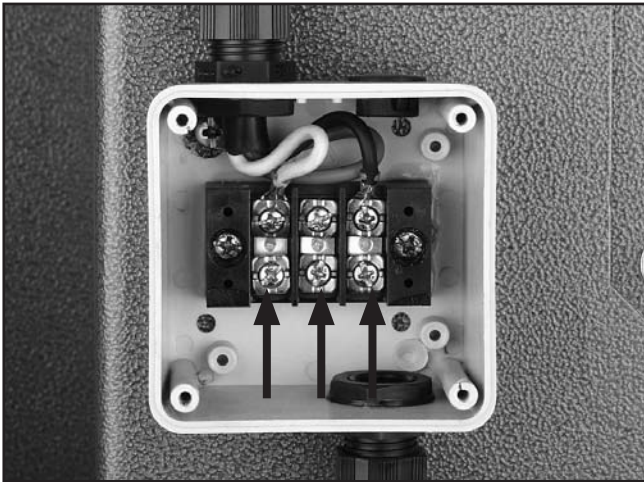
Figure 47. G0591 main terminal box.
