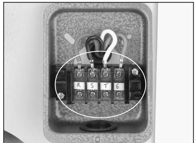
Figure 28. Main terminal located inside the electrical wiring box, on the outside of the cabinet.
